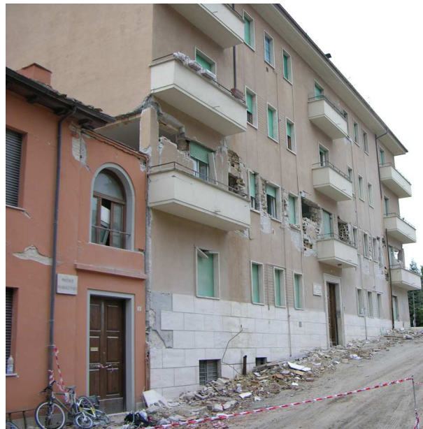
Figure 1: Damage of a four-story conventional building due to pounding with its adjacent two-story building, during the L'Aquila earthquake in Italy, in April 2009 [5].
