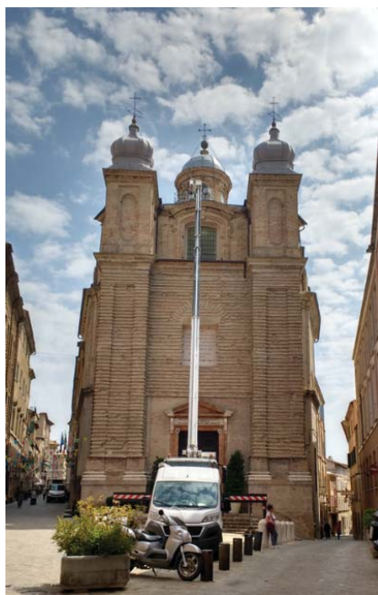
Figure 1 San Filippo Neri in Macerata nowadays during the execution of the AVT
