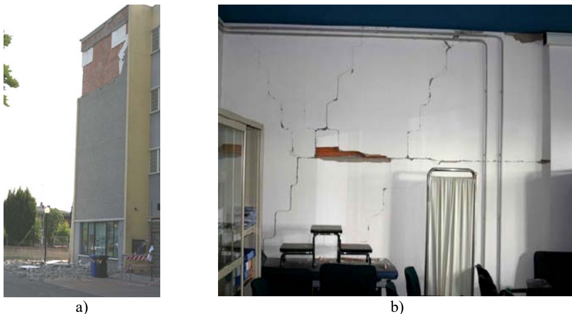
Figure 1: Example of damage to Service Centre: a) collapsed infills and b) cracked partitions .
