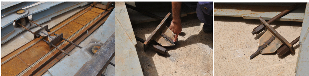
Figure 7: Fuse device before and after failure.
