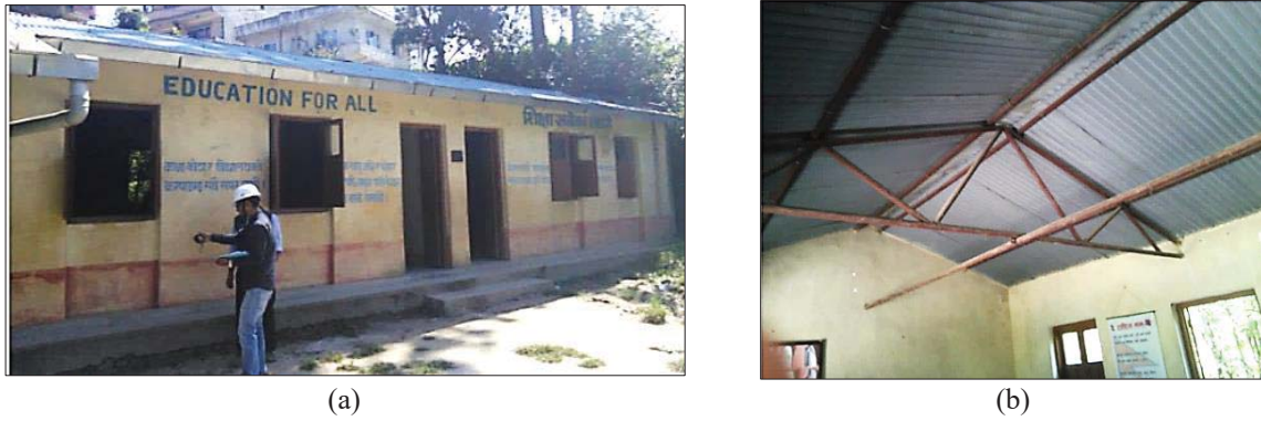
Figure 4: Photographs representative of the case study URM school building: (a) outside front view and (b) Inside view showing the short walls with gables and light steel roof structure. (Image Copyright: The World Bank)
