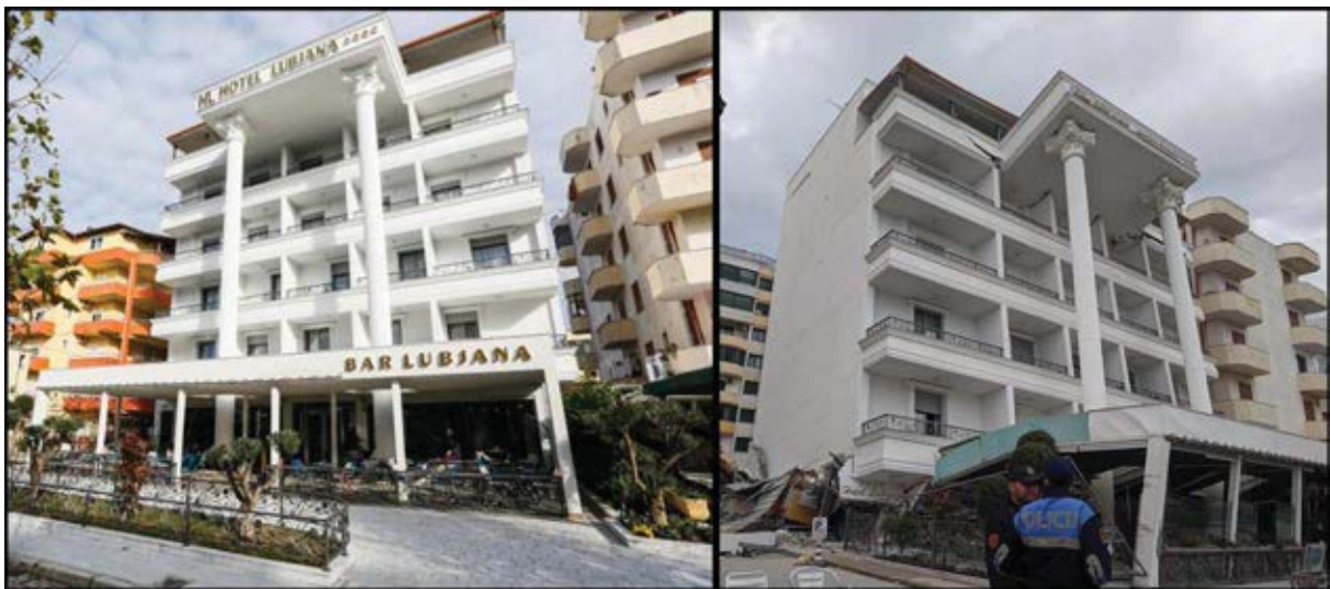
Figure 14: Collapsed Lubjana Hotel in Durrës (Left photo: [29], Right photo: courtesy of C. McKenney [28]).
