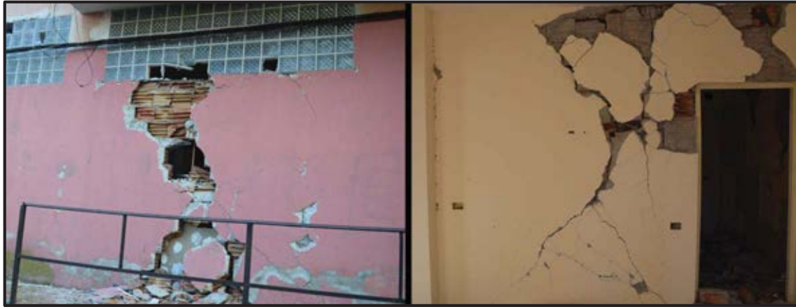
Figure 9: Infill in-plane failure.
