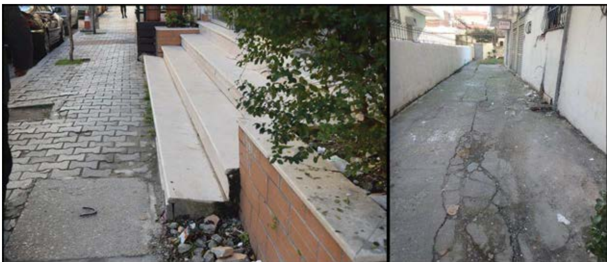
Figure 15: Soil settlement in buildings.
