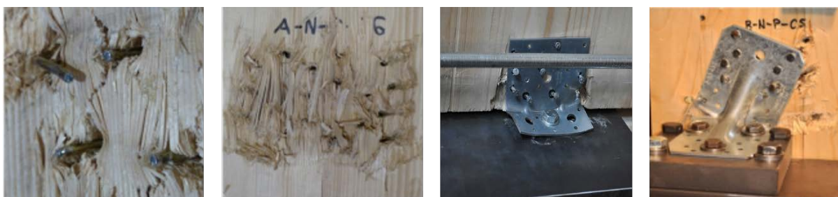
Figure 1: Typical damage in connections made with hold-downs and angle-brackets.
