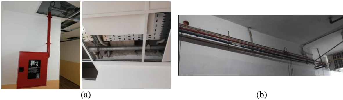
Figure 2: Fire-fighting system and (b) heat water piping system tested.
