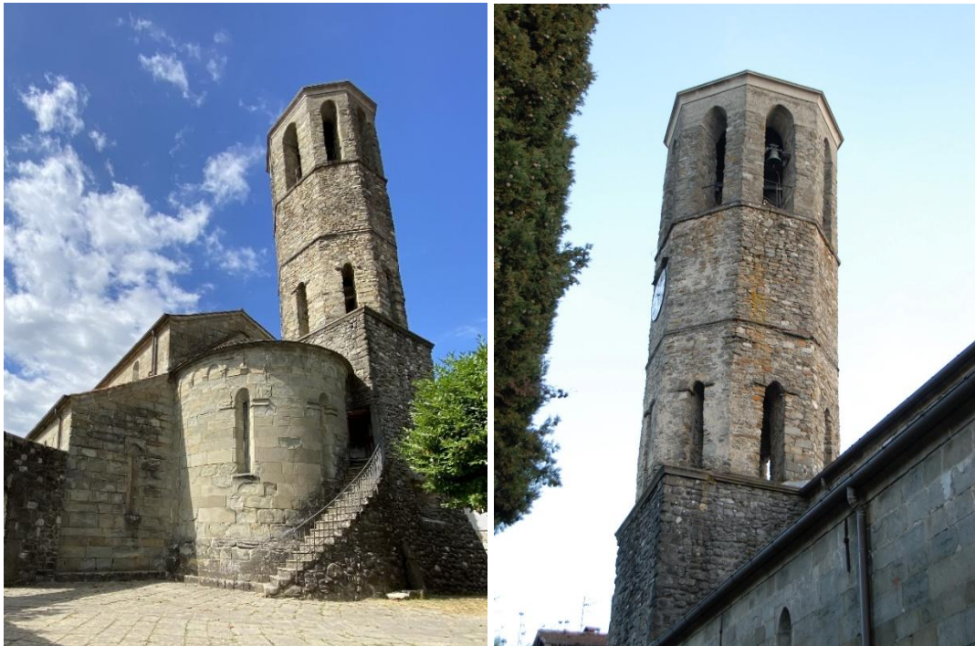
Figure 1: The bell tower of Pieve San Lorenzo, Minucciano: view from the apse and from the naves.
