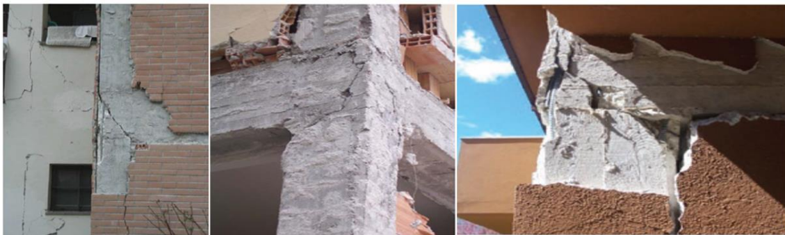
Figure 1: Damaged RC beam- column joints with diagonal cracks following an earthquake [16]
