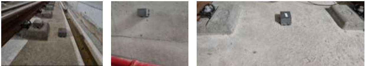
Figure 5: Photographic record of the sensors used for vibration measurement at the track and tunnel wall level.
