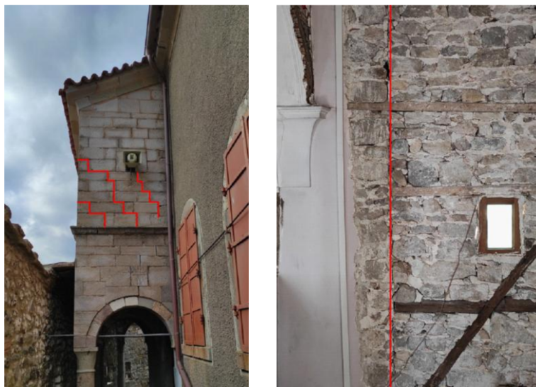
Figures 5 and 6: Cracks at the external layer of the masonry of the gallery. Insufficient connection and detachment of the gallery from the main temple.
