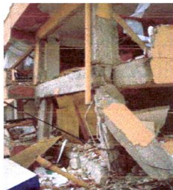
Figure 1: Beam-Column Joint Failure in RC Buildings Turkey, 1999 [15].
