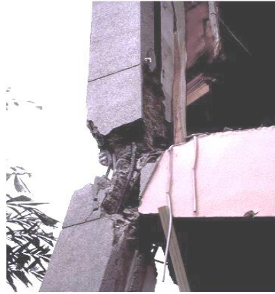
Figure 2: Joint Failure due to Inadequate Detailing Taiwan, 1999 [3].
