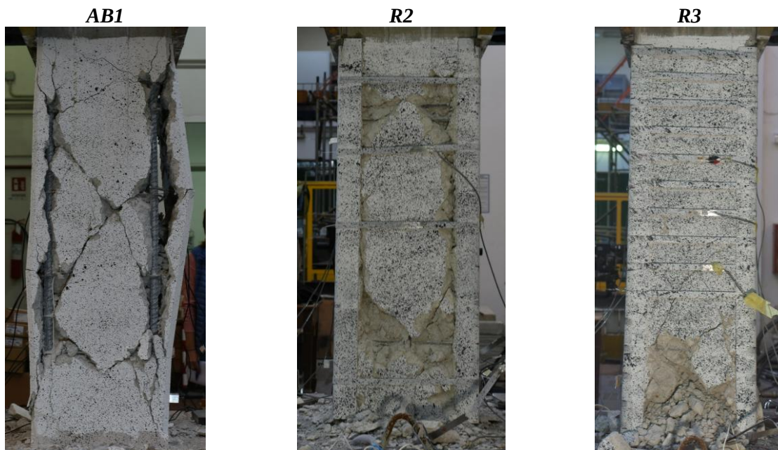
Figure 8. Damage state at the end of tests.
